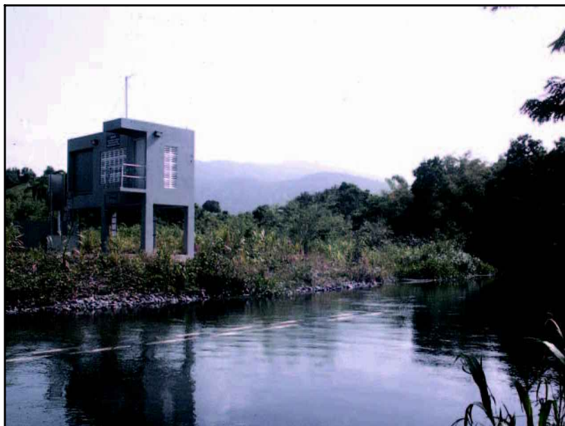
Figure 5. The in-channel withdrawal structure located on the Río Mameyes, Puerto Rico. Water is pumped from the submerged stainless steel risers to the pumphouse on the bank. Photograph: James March.
